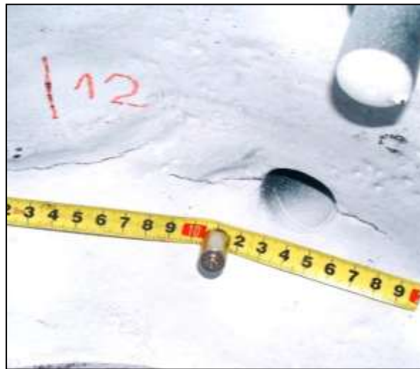
Left Image: Cracks on the inner surface of the casing exposed to the high-pressure steam flow
