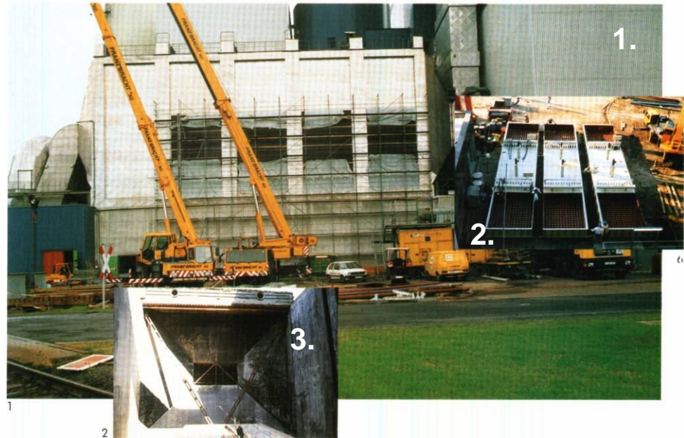
Pic 2 Pre-mounted clean gas chamber
