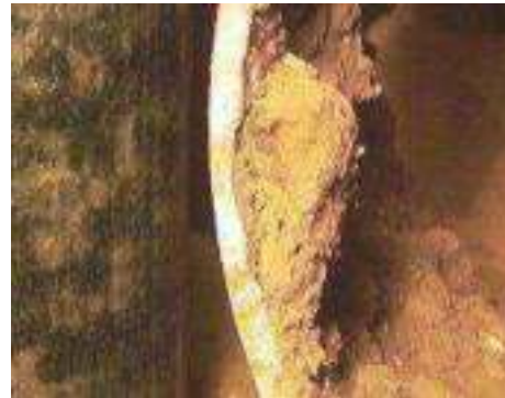
Under deposit Corrosion
